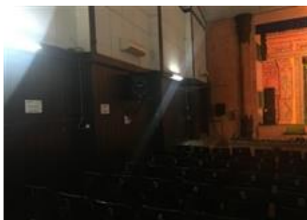
Gambar 11: Peredam Dinding Auditorium RRI Surakarta
