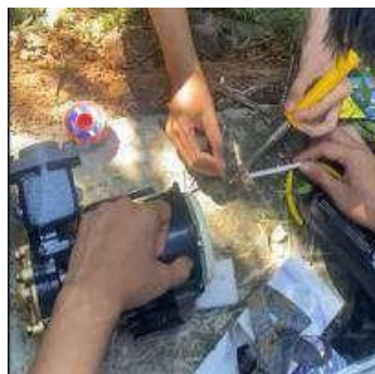
Gambar 2. Instalasi Sensor Digital Timer
